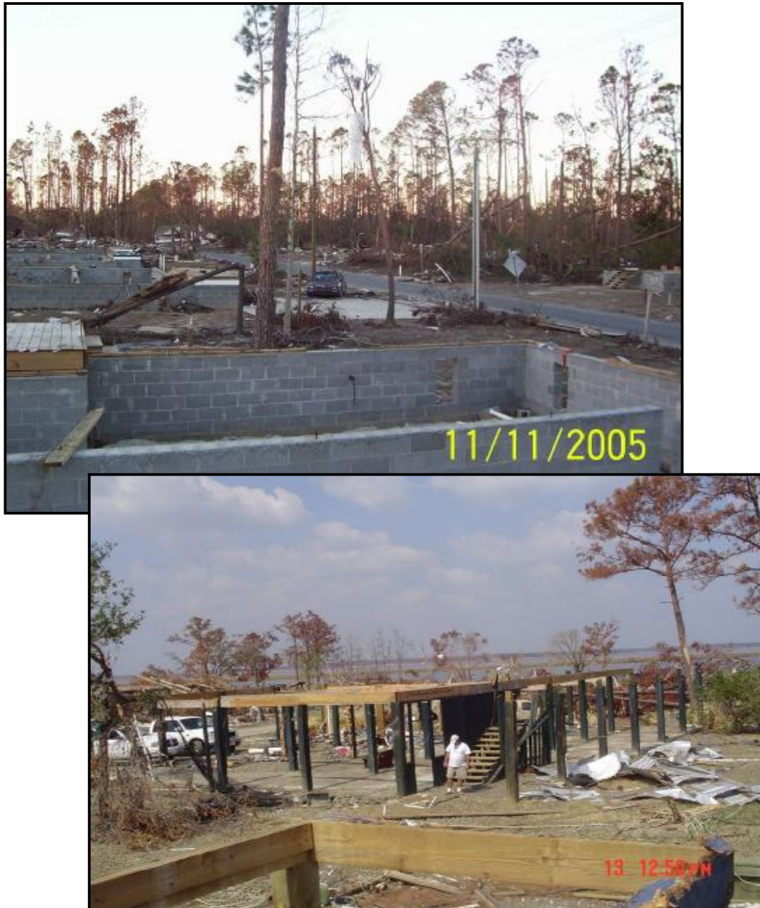
Figure 6: Typical views of devastation along the Mississippi coast caused by Hurricane Katrina. Determining the extent of wind damages prior to the storm surge sweeping through these sites was a daunting task for the structural engineer.
