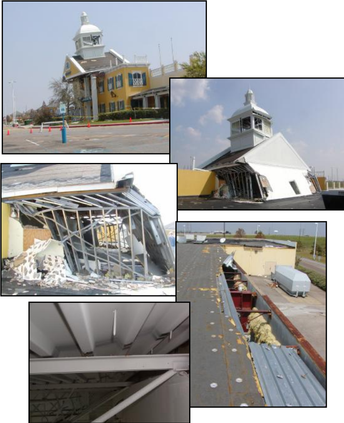
Figure 10: Series of photographs that documented damages to the shopping mall. The partial collapse of the elevated roof structure was attributed to construction defects (inadequate bracing / unstable construction) whereas the removal of localized portions of roof deck occurred at the perimeter due to the failure of puddle welds.
