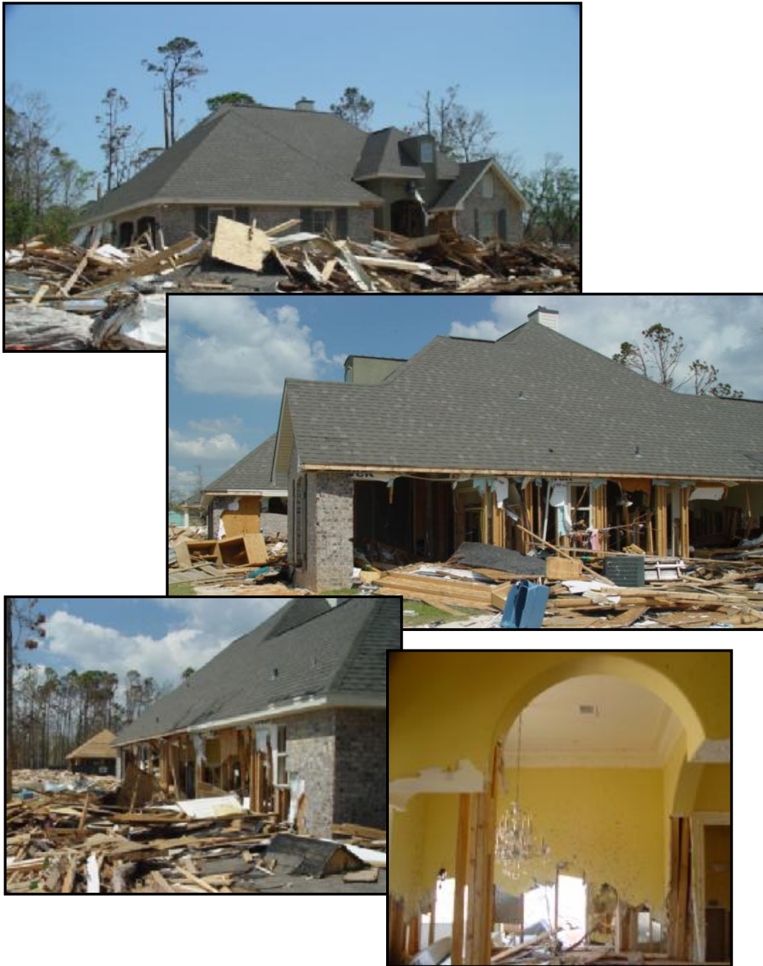
Figure 8: Series of photographs that documented damages to the house. Note that minimal damage was present to the roof covering, while severe damages were on the lower part of the structure. This was a good example of typical damages caused by the storm surge from Hurricane Katrina.
