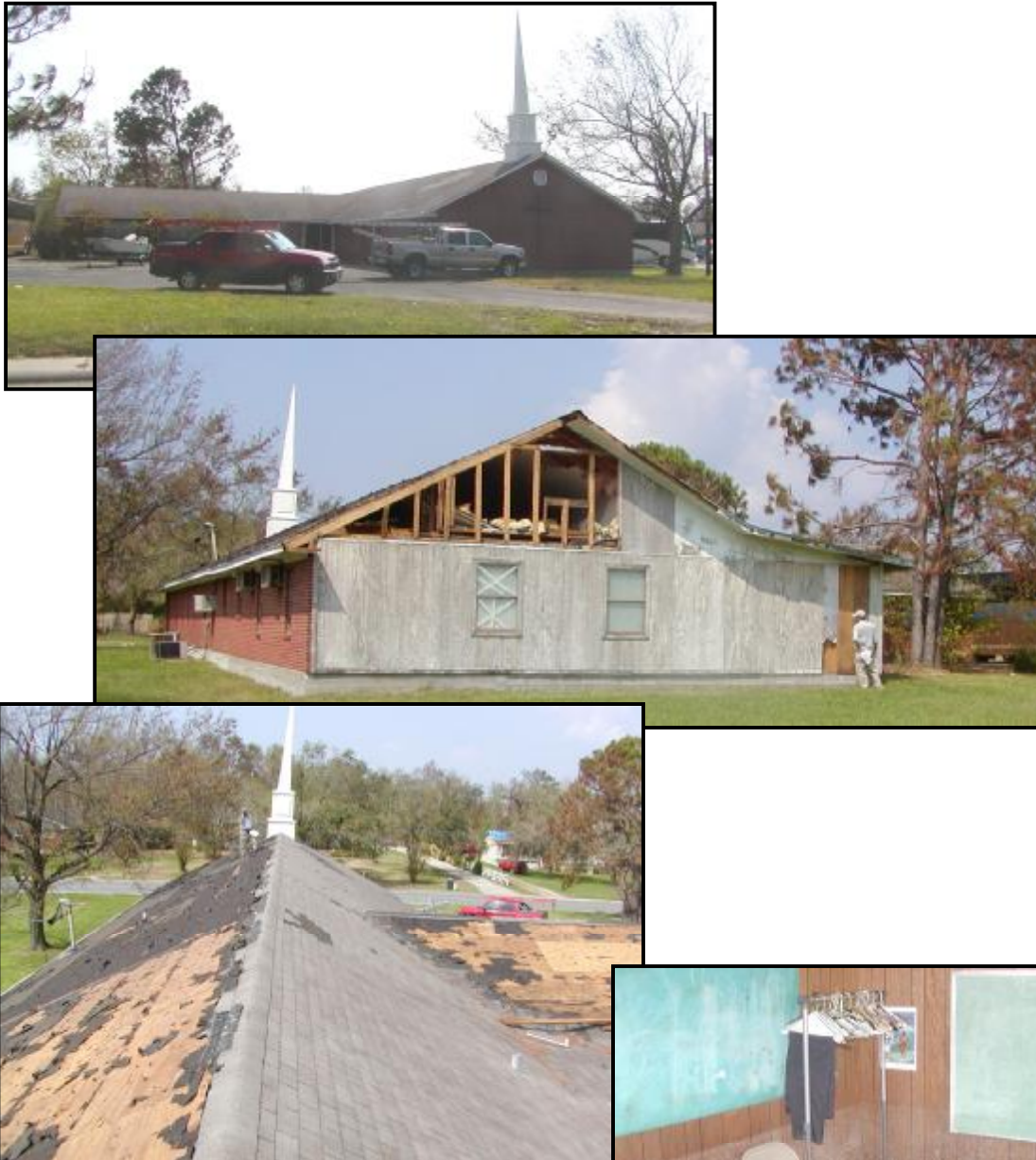
Figure 7: Series of photographs that documented damages to the church structure. In this example, the forces from wind caused the majority of structural damages, while the surge caused extensive water damages to the interior. This is a good example of typical wind damages caused by Hurricane Katrina.
